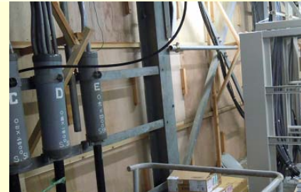
<Air-conditioning is newly installed and plywood is replaced by a complete wall to ensure the effects of air-conditioning>
