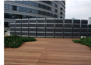
Solar power generation system
