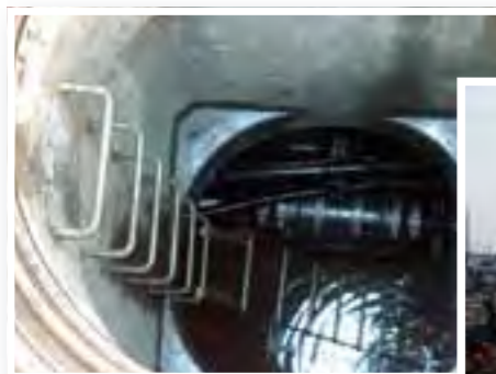
Manhole filled with water (Ofunato City, Iwate Prefecture)
