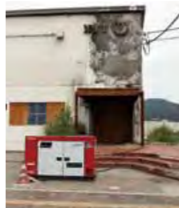
Emergency generator deployed at the Otsuchi Building (Otsuchi Town, Iwate Prefecture)
