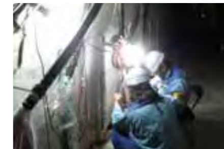
Connecting lines under lamp light inside an exchange building
