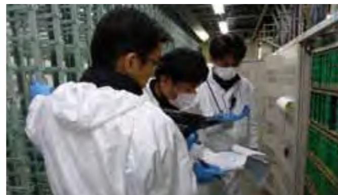
Our employees were allowed four hours to complete all necessary work. There were some difficult aspects, but the work went smoothly and we managed to restore functions in the given time.
