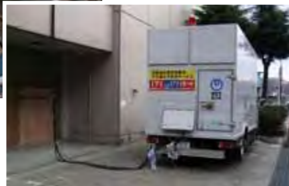
Power supply vehicle supplying electricity to the Miyako Building (Miyako City, Iwate Prefecture)
