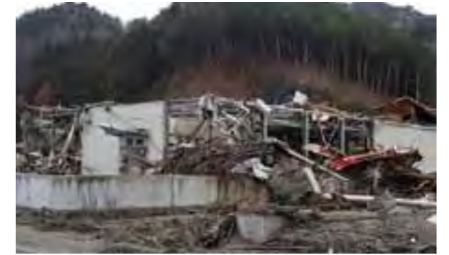
The devastated building
