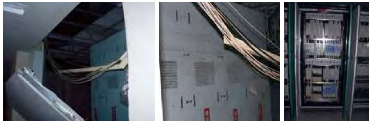
Seriously damaged ground floor power supply equipment
